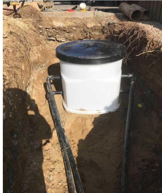
Borehole connection manifold in position.
