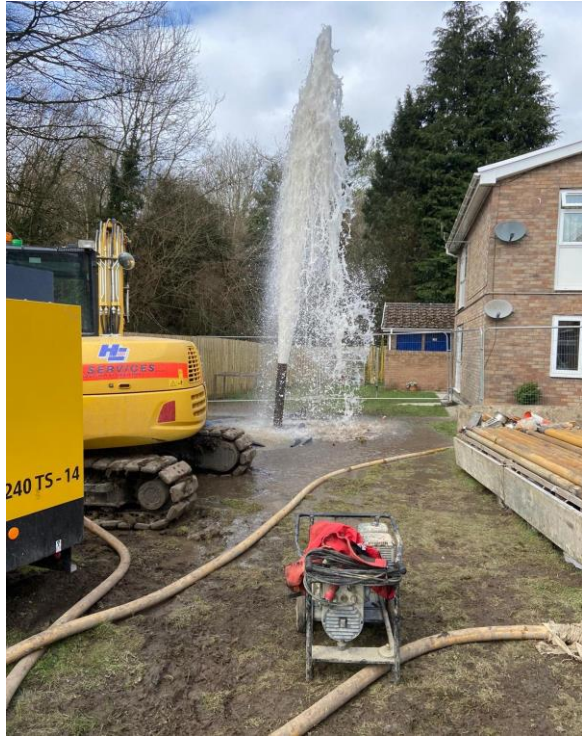
An example of fractured ground with a substantial water strike, very rare but does occur.
